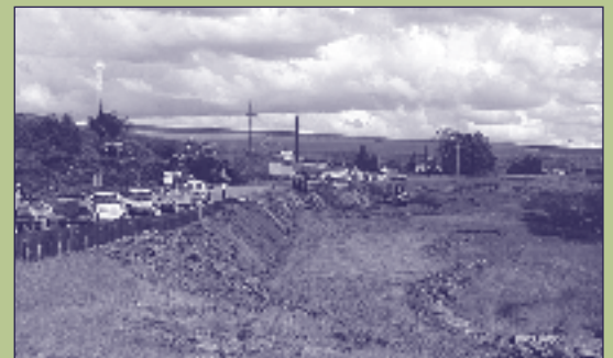
Excavation on the southern end of the Top of Lewiston Hill to Genesee Project.
